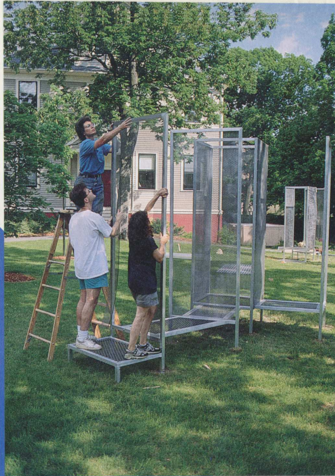
Bunting Institute sculptor Beth Galston and student interns install “BodyHouse: Outdoor Environmental Sculpture,” on the grounds of the Institute in May.
